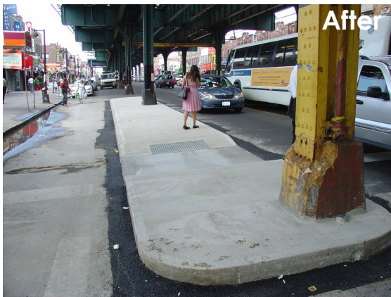
After: 86th Street and Bay Parkway, Brooklyn, NY. Source: New York City Department of Transportation
